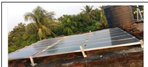
Fig. 3- Solar Cell in the roof top of the building for experimental set up
