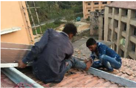
Figure 2 (d) Roof top installations exposes workers to risks of fall from heights and injuries from sharp edges of solar panels/frames
