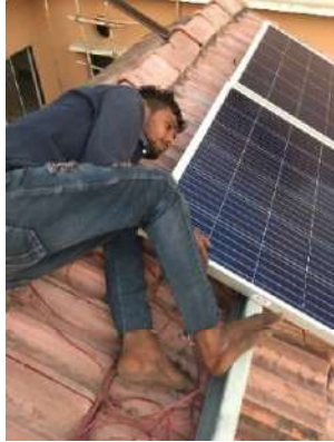
Figure 2 (c) Work in confined spaces, awkward postures and lack of PPE are potential hazards
