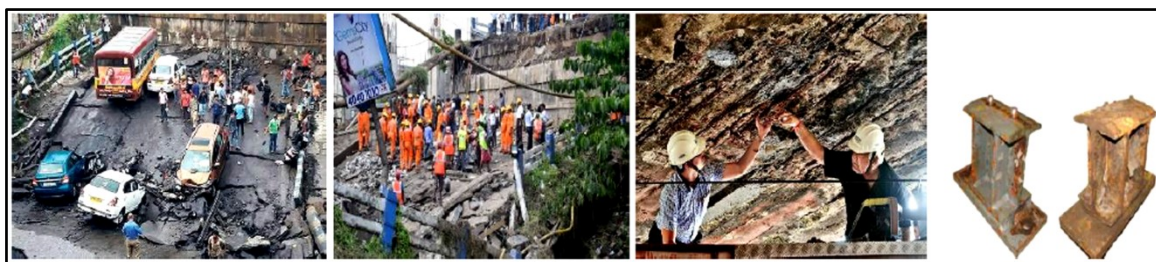
Figure 1 (a)-(b) Catastrophic failure of bridges, (c)-(d) Distress in bridge deck slab and bearings [4]
