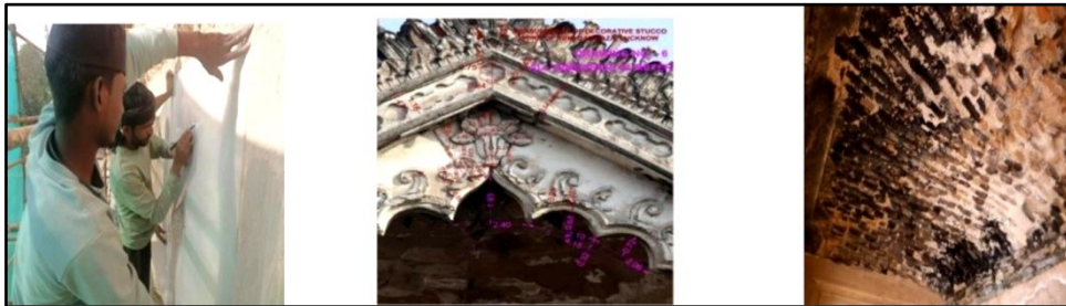
Images 2A, 2B & 2C Proper Documentation like photo, video, drawings, site plan, sectional plan of each and every part of structure and study the causes of structural problems
