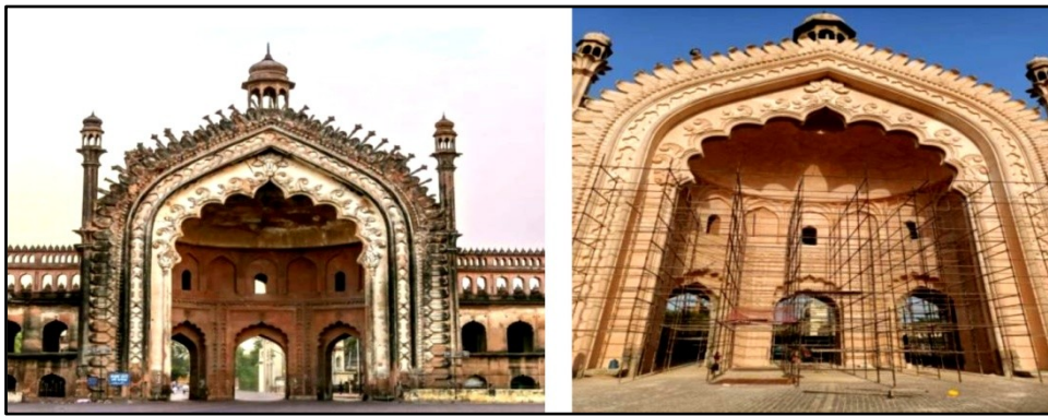
Images 5A & 5B Rumi Gate main structure before, during and after major conservation works
