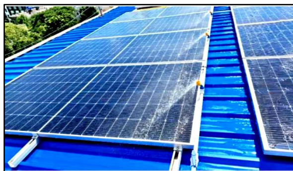
Figure 1 Semi-automated cleaning under progress of the solar PV power plant
