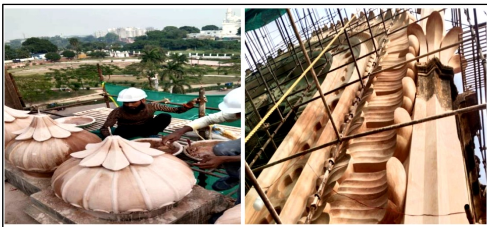
Images 3A & 3B Stucco work, design moulding work, highly rich intricate plaster work in traditional lime mortar with natural adhesives
